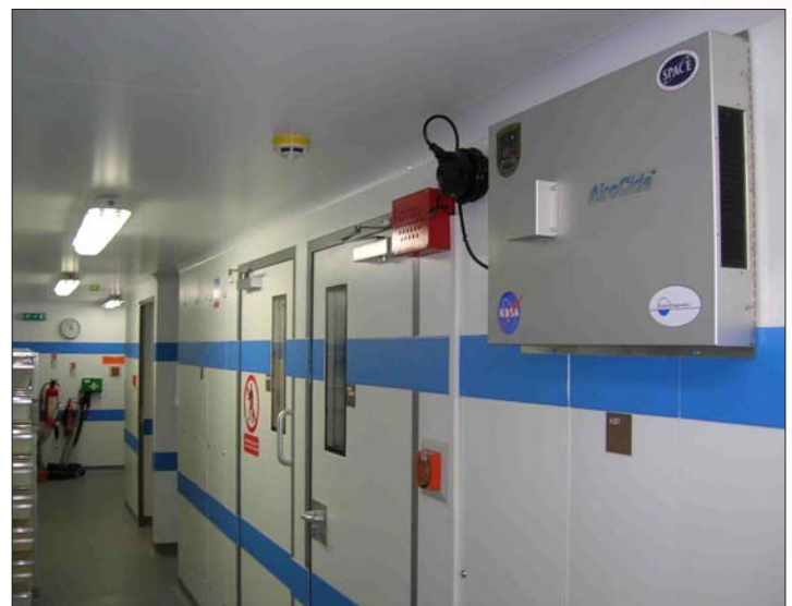
Airocide® unit positioned in corridor
